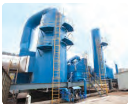
VOCs Purification System
