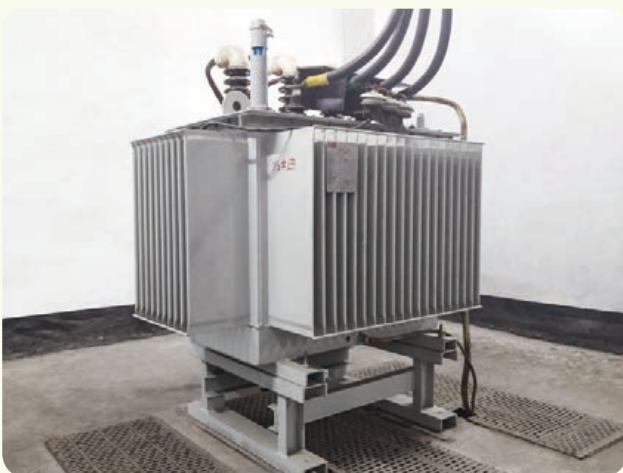
Oil Immersed Transformer
